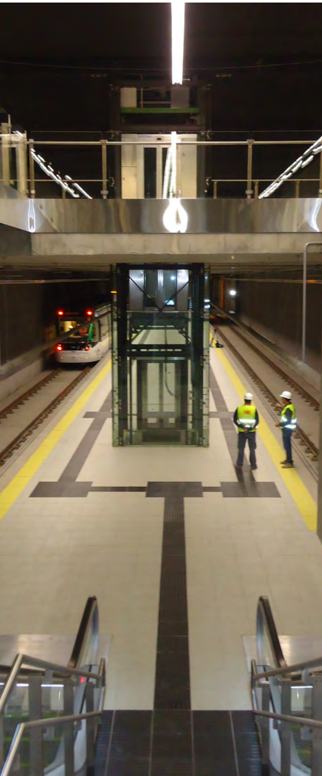
Malaga Metro installations
